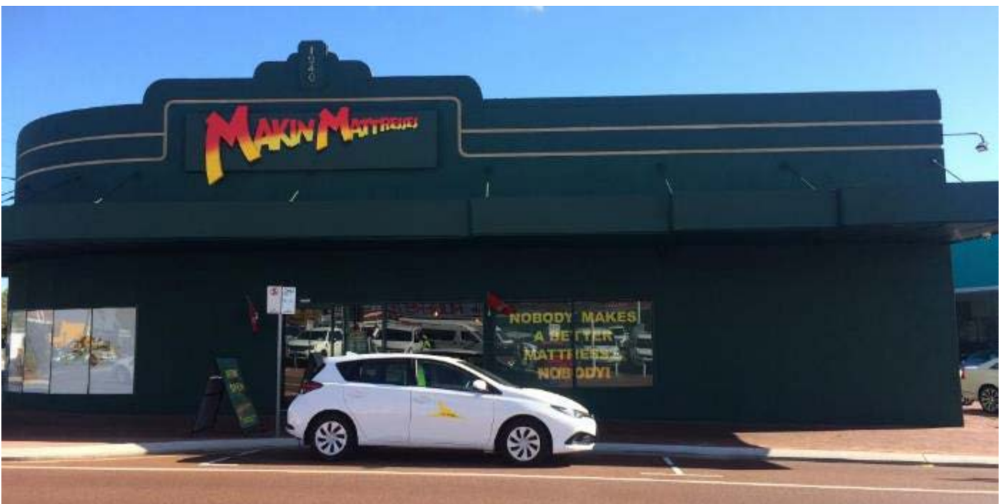
Figure 10: Blocked up windows to facade and covered up name panel
