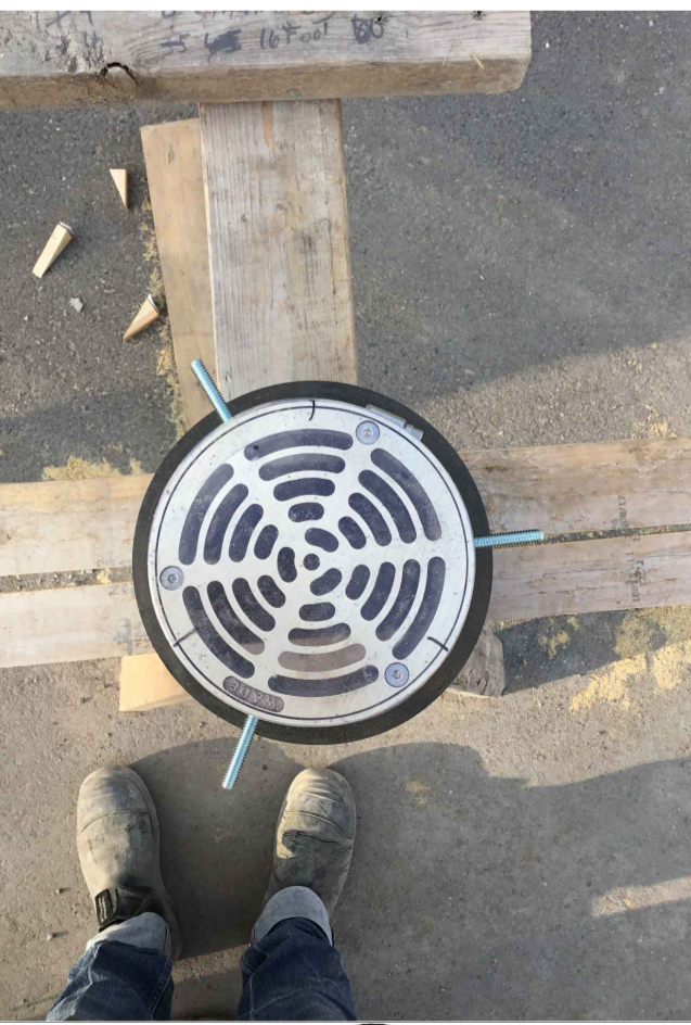
ENSURE ADEQUATE CONNECTION TO CONCRETE SLAB / TO PREVENT SINKING OF DRAIN RIM. SEE PIC
